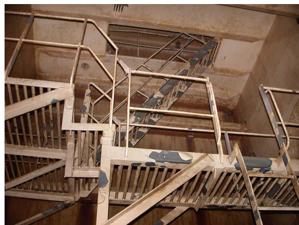
Photograph 2. Corroding zinc on the PMA itself is removing the paint.
